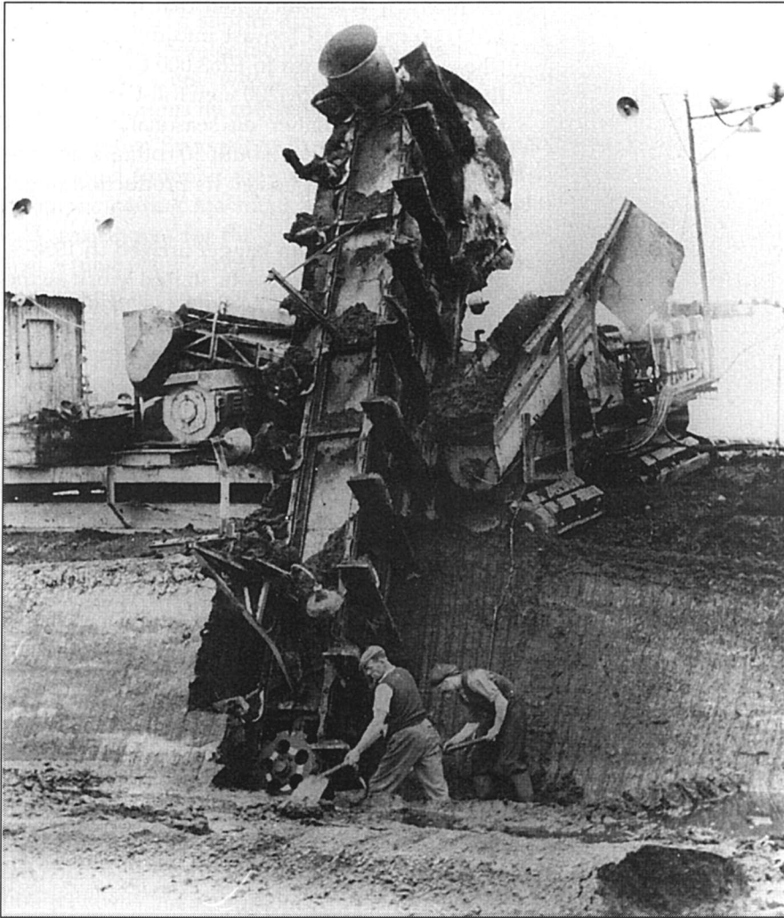
Figure 4.3: Bagger in action. The automatic excavator cuts a 2m wide bank of peat to a depth of 3m. The macerated peat is fed out onto a 54m spreader arm in a continuous 'sausage', and is deposited in parallel rows where it is cut by discs. The diagrams show the general layout and design of the Wielandt and Dolberg machines.
